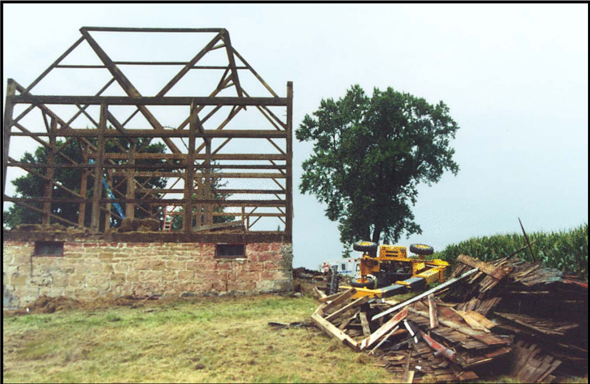
Photo 2 – View from the north side of the barn, showing the barn structure, the overturned forklift, and the broken rafter section lying next to the pile of discarded roofing.
